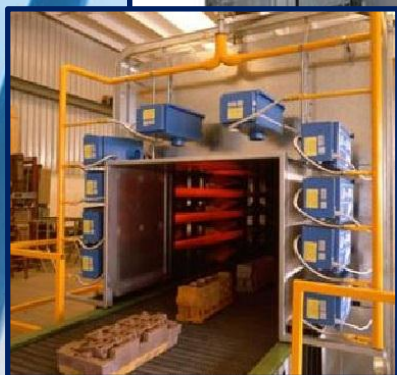
Module of power regulator M25 in industrial dryer furnace
