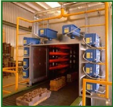
Module of power regulator M25 in industry drying oven
